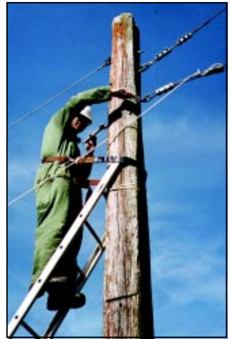
Brian Miller, ZL1AZE, making a few repairs to the lower end of the sloping V antenna.
