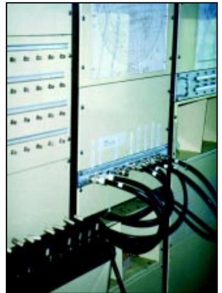
The antenna terminal room.
